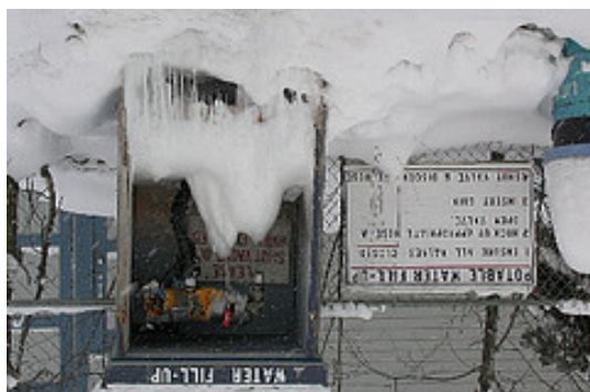
Today's journal features - water fill up and gas for less
